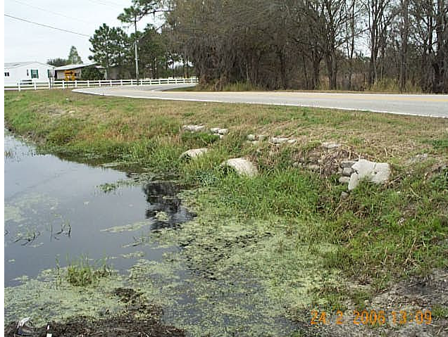
Looking east at the downstream side of the culverts under Patterson Road from the west side of the street.
